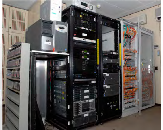
Server and backup infrastructure for the WIS-network
