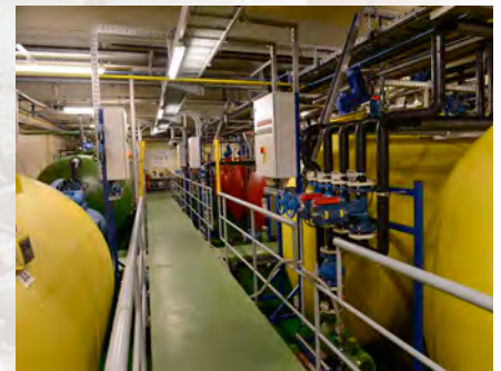
Facility for the processing of radioactive contaminated sewerage
